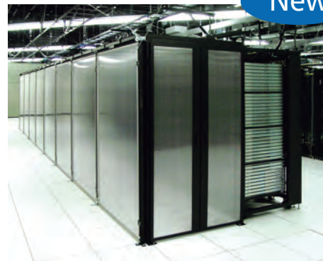
Aisle Containment, pg 36-37
